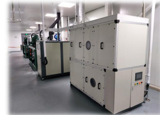
Rotary dehumidifier (Swedish imported brand)
