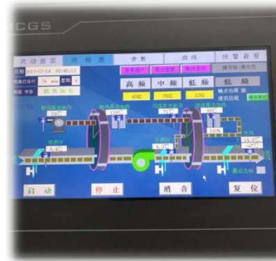
Dehumidification control screen
